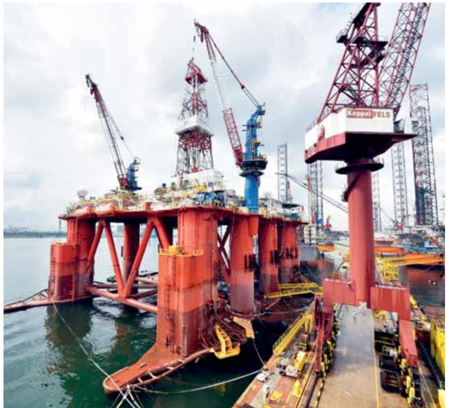
Semisubmersible drilling rig Hakuryu-5 made a repeat visit to Keppel FELS in November 2015 for repair and refurbishment work
